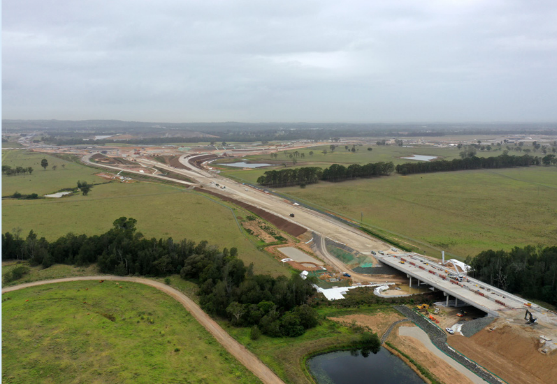
Aerial view of construction of Cosgorves Creek bridge and the Airport Interchange looking east
