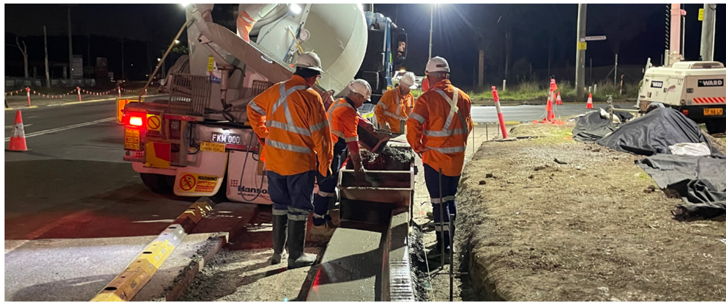
Extrusion of kerb on southwest corner of Devonshire Road and Elizabeth Drive Intersection
