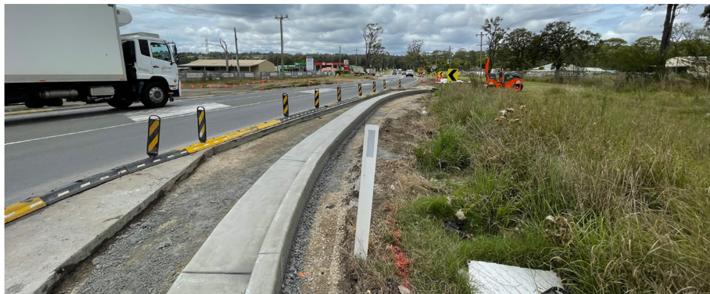
Completed kerb on southwest corner of Devonshire Road and Elizabeth Drive intersection
