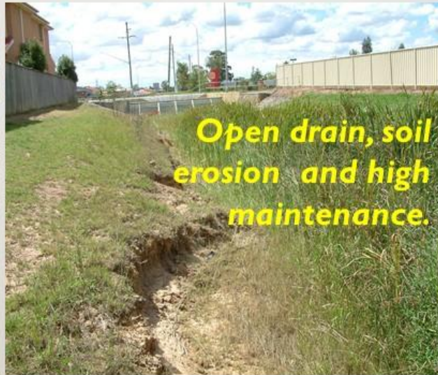
High maintenance, requires regular rubbish removal.
